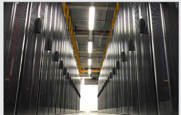
Increasing data speed in data centers poses cable management and space challenges
