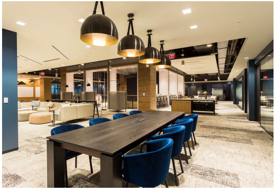
FIGURE 2: PoE pendants/light fixtures.
